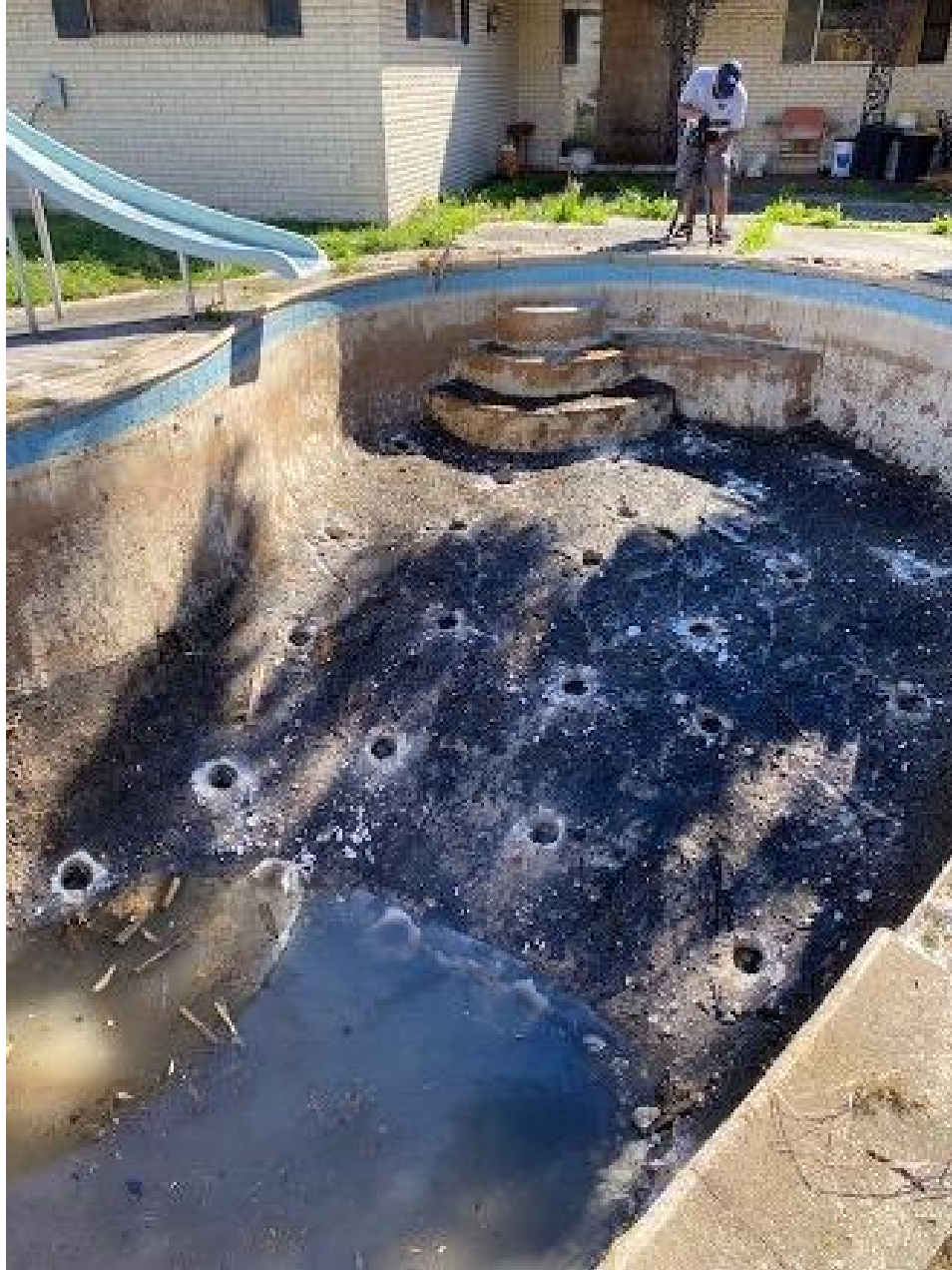
The pool at 5700 Vicksburg was a blighted, mosquito-ridden nuisance for 17 years. Last month, Code Enforcement drained and filled the unsecured pool.
